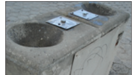
The score for this Drinking Fountain at Orchard Beach was impacted by a loose panel and graffiti.
