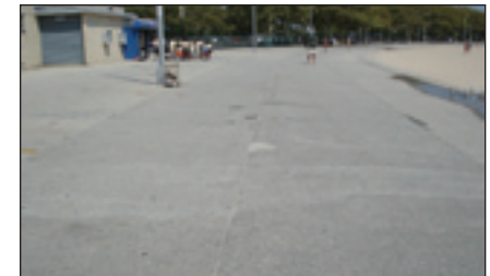
Aside from small cracks, the concrete Pathway at Manhattan Beach is in good condition.
