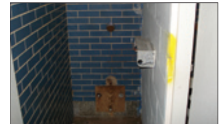
Damaged and missing equipment in Midland Beach's Bathrooms resulted in a low score for this feature.
