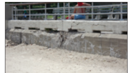
The wall bordering the shoreline at Orchard Beach is deteriorating and unsafe.
