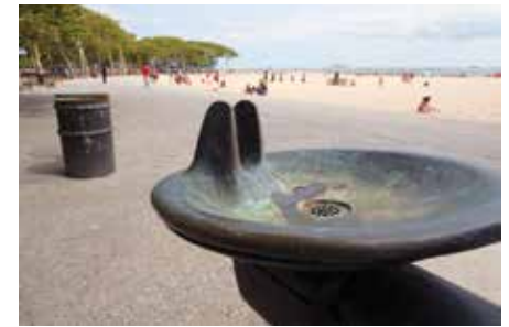
Drinking fountains across the city's beaches would benefit from frequent plumbing work
