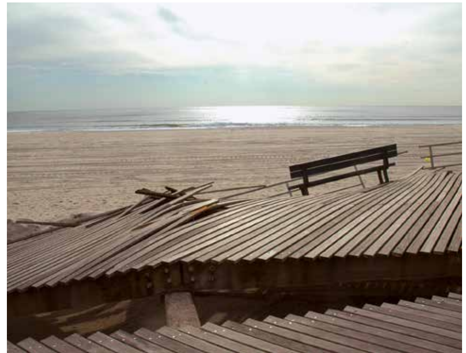
A damaged section of boardwalk at Rockaway Beach, Queens.
