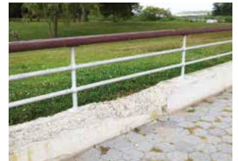
Deferred maintenance and storm damage have contributed to the deterioration of the Orchard Beach Ship's Rail
