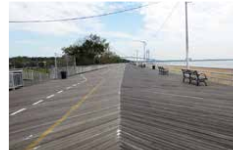
South Beach's boardwalk, with the Verrazano-Narrows Bridge in the background, is in very good condition
