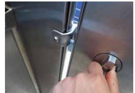
Many bathroom stall doors are damaged and do not lock
