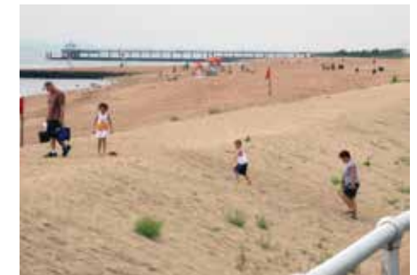
Protective dunes have no signage or clear access points, leaving the structures vulnerable to beachgoer traffic
