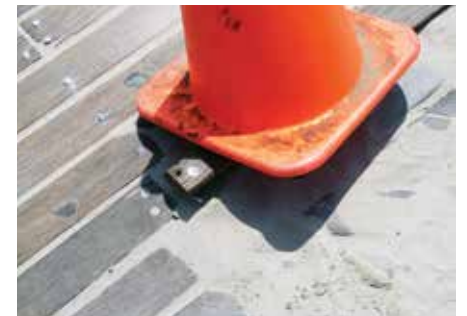
A broken boardwalk plank and sand create a trip hazard on a pathway
