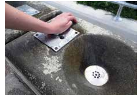
Pressure at this drinking fountain is too low to allow use
