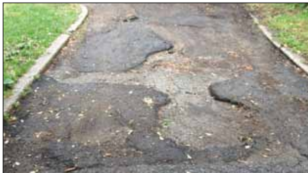
Deteriorating asphalt was a common problem on park pathways.
