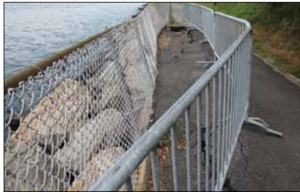
Dangerous sinkholes on the waterfront pathway
