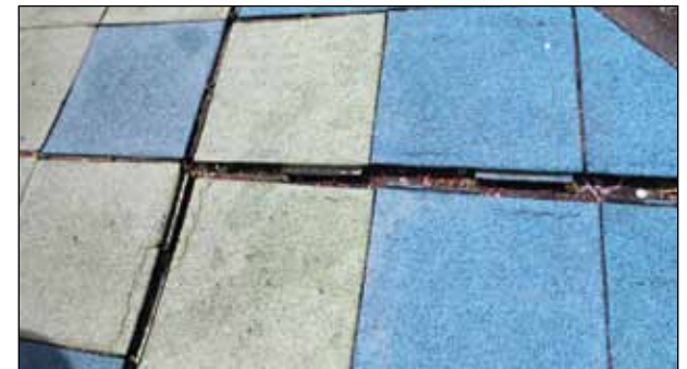
Deteriorating or splitting safety surfacing was the most common problem in playgrounds.
